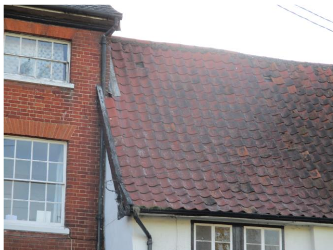
Photograph 3 Building within the village showing potential bat roost features: missing roof tiles and lifted lead flashing.
